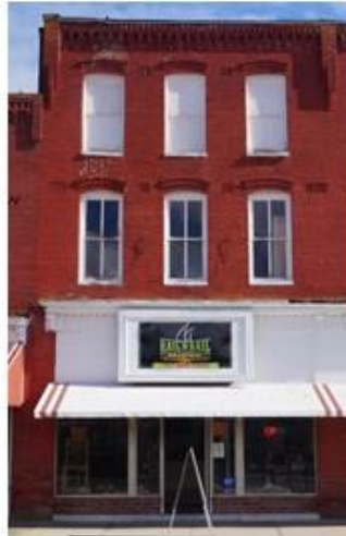
P61 – Rail & Sail Seafood, 18487 Dunne Ave. Economic Blight: No; Physical Blight: Yes but structurally sound
