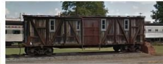
P79 – Railway Museum Historic Box Car, 18444 Dunne Ave. Economic Blight: No; Physical Blight: Yes but structurally sound
