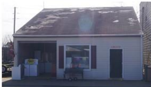
P19 –Appliance Repairs, 24286 Bennett St. Economic Blight: No; Physical Blight: Yes with potential structural issues
