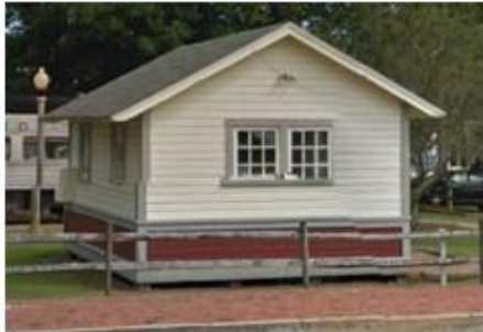
P75 – Railway Museum Historic Maintenance Tool Shed, 18444 Dunne Ave. Economic Blight: No; Physical Blight: Yes but structurally sound
