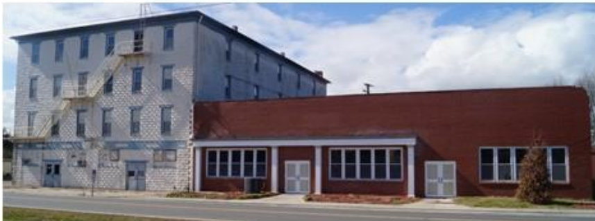
P03 – Former T-Shirt Factory, 18554 Cassatt Ave. Economic Blight: Yes; Physical Blight: Yes with potential structural issues
