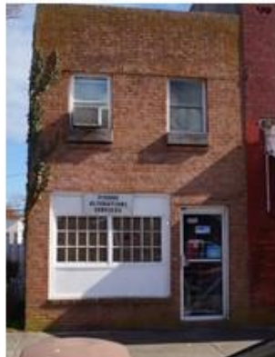
P59 –Pierre Alterations Service, 18483 Dunne Ave. Economic Blight: Yes; Physical Blight: Yes but structurally sound
