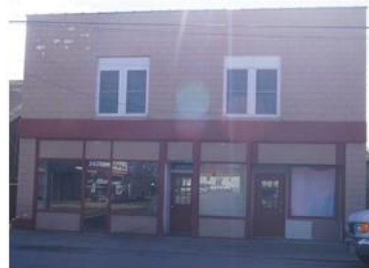
P18 –Vacant Store, 24280 Bennett St. Economic Blight: Yes; Physical Blight: Yes with potential structural issues
