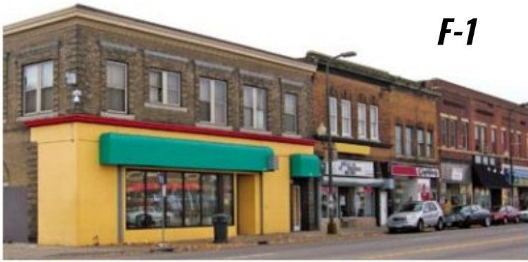
BEFORE Covering brick with another material, like the yellow boards in this photograph, is discouraged.
