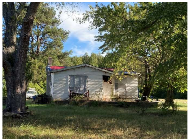
Figure 6: Several structures in dilapidated condition were observed, including those with missing windows and roof damage that may not be rebuildable.
