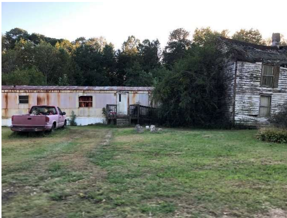
Figure 17: When the main structure fails, some residents bring a mobile home onto the property. Consultants also heard of this approach during the public meetings.
