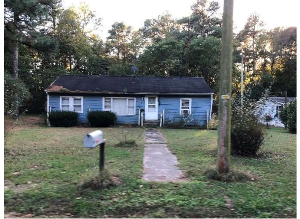
Figure 16: There are examples of homes in poor condition. Aside from issues with siding and windows, there was degradation with roofing. In this example, there are missing shingles on the left and what appears to be a warped roofline.
