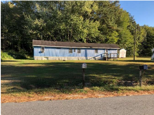
Figure 13: Consultants counted seven single-wide homes and other type of mobile home options. While some are in fair condition, others have issues like sagging rooflines.
