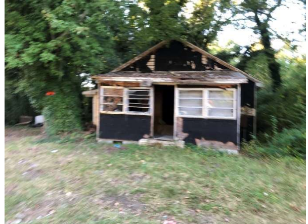
Figure 2: Housing conditions tend to decline farther to the western end of the neighborhood. There are also a couple of dilapidated homes that appear to be vacant.
