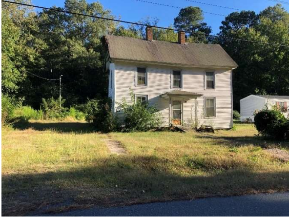
Figure 11: There are several structures in poor condition. A sagging roofline indicates serious structural issues that require expensive renovations. In these instances, demolition and replacement may be more affordable.
