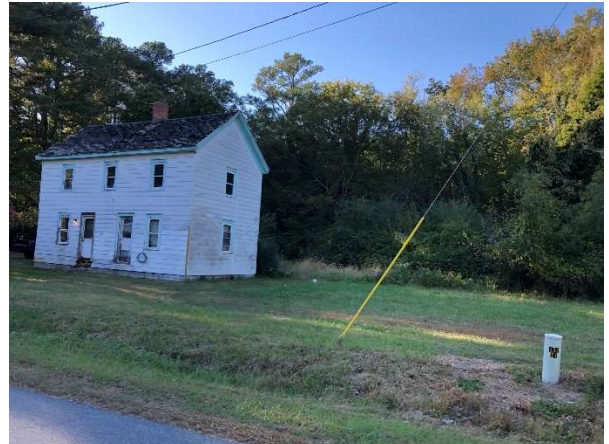
Figure 14: Many homes had wear and tear with siding. Others had more serious issues, especially with roofing. In this example, the roof shingles are deteriorating.
