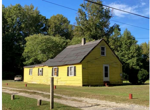
Figure 4: Houses like this example with an unshingled roof require urgent repair to remain viable.
