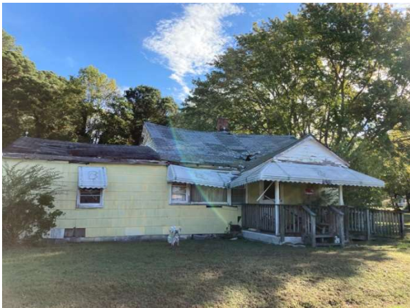
Figure 9: Several abandoned homes were noted with severe structural failure such as collapsed roofs. These units are unlikely to be repaired and rehhabited.
