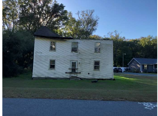
Figure 12: There are several dilapidated and blighted properties on Bayside Road. Without proper resources to repair minor issues, structures can rapidly deteriorate.
