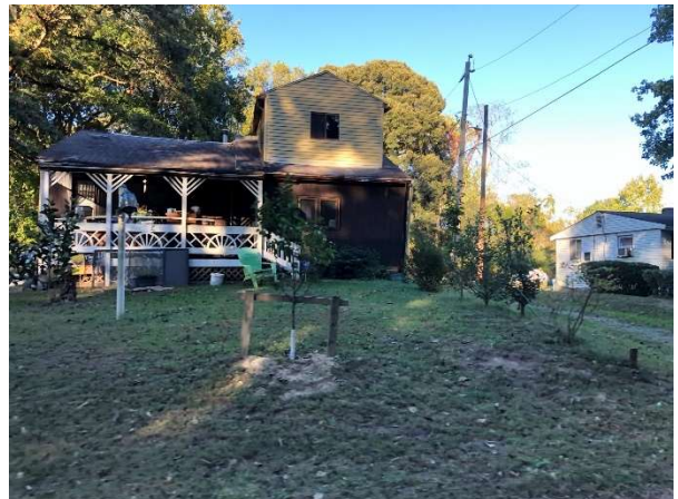
Figure 8: Some homes in fair condition may soon fall into poor condition without property maintenance and repair. In this example, there are missing shingles to the left that will require a more expensive reroofing effort.
